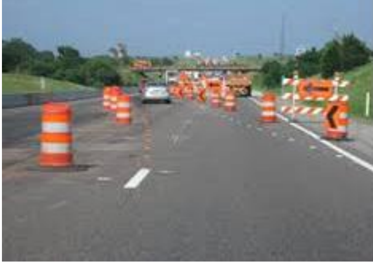
Figure 3-7 Channelizing Device: Barrels
